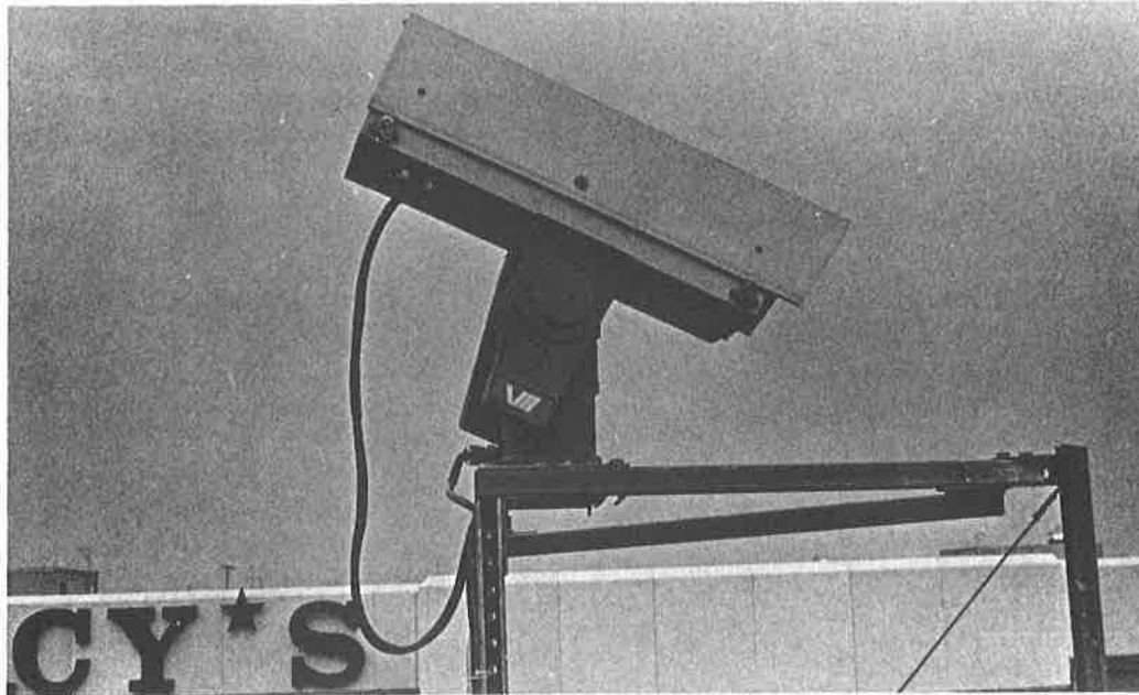
Heart of security tv at Kings Plaza is the monitoring console (far left) manned round the clock seven days a week. Cameras are spotted such places as in camera housing on ceiling inside center (upper left), or outside (lower left) to cover such areas as receiving docks. Outside camera can operate at low light levels, thus protect at night as well as in day.
